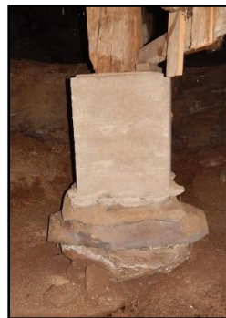
Old pier resting on stones.
